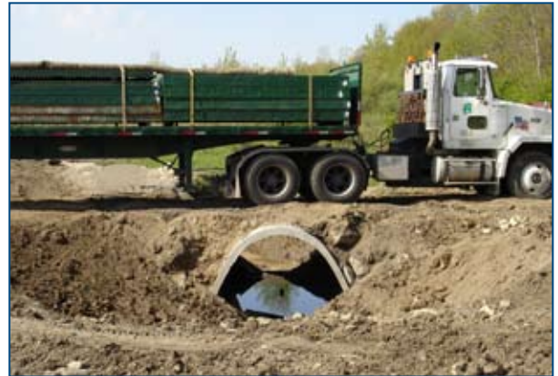
Design Loading - Full-scale testing verified design methodology and safety factors for AASHTO loading.
